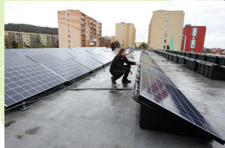
PV power station on a school
